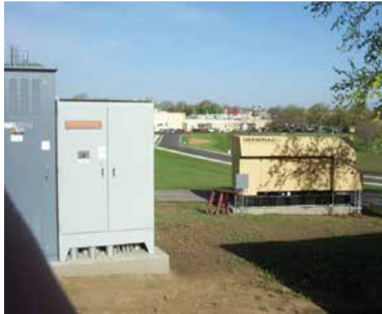
BIVI's Gemini gensets backs up their maintenance and boiler building.
